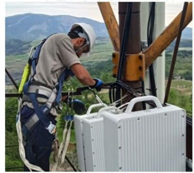
Mobile Base Station
