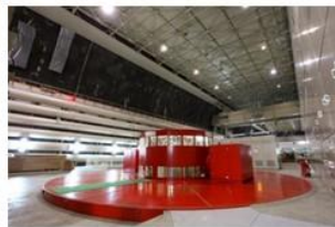
Pumped Storage Power Plant as Countermeasures for RE introduction
