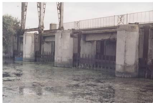
View of the available main water receiver manhole of Lower Shirvan Canal from the below part
