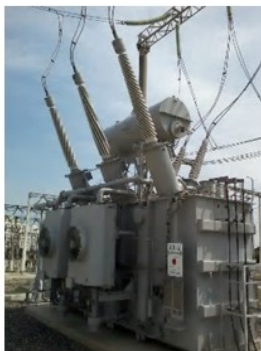
Mushviq substation (grant, 2006)
