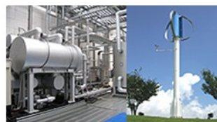
Environment (Air Condition)
